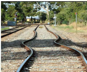
Heat can make rails buckle, as seen in this picture, causing trains to derail.
